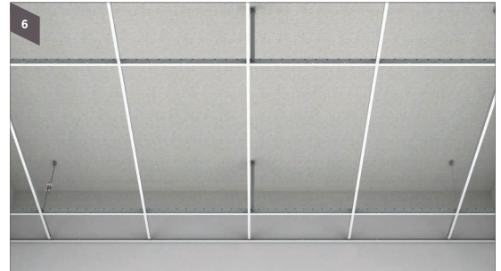
Insert the long cross tee to main tee in place for 600x600 module
