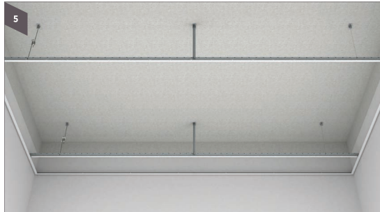
Fix the main tee at 1200 mm spacing and lay it on the wall angle.
