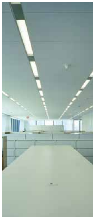
Logix Integrated Ceilings
