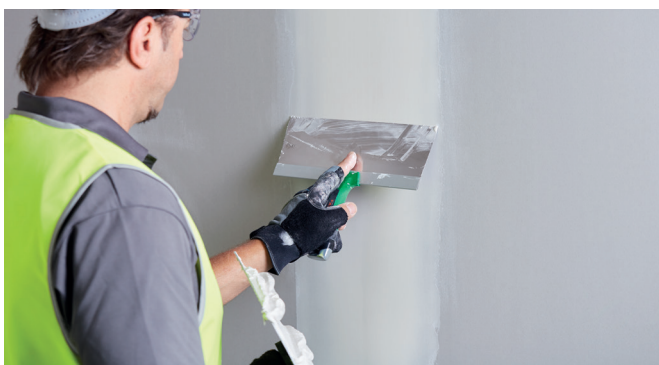
Step 5 For second and finishing coats apply as per tapered or square edge joint and finishing application
