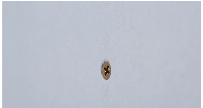
Good fixing of screw or fastener into plasterboard
