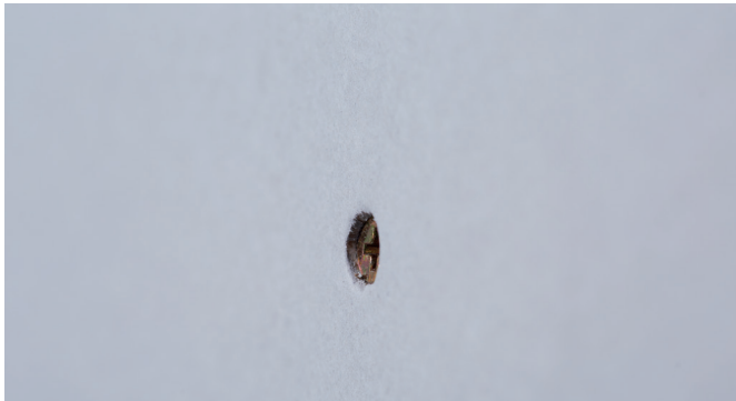
Poor fixing of screw into plasterboard
