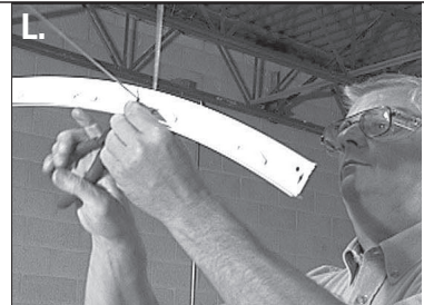
L. Hang the flush-cut end of the main tee from the ceiling at the elevation and location specified on your architect's plans or by scaling from a working drawing.
